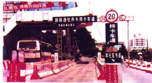
There are now 23 electronic tolling locations, in or around Foshan City with 36 electronic toll collection readers spread between them
